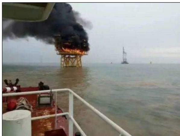
Figure 3 – SPIC Binhai North offshore substation fire [10]
